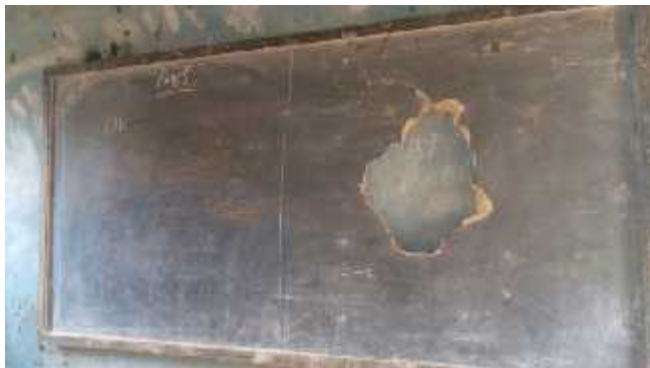
Figure 4-1. Above picture is taken on 4/4/2017. It shows the blackboard damaged in a classroom which is shared by 8th and 4th grade.
