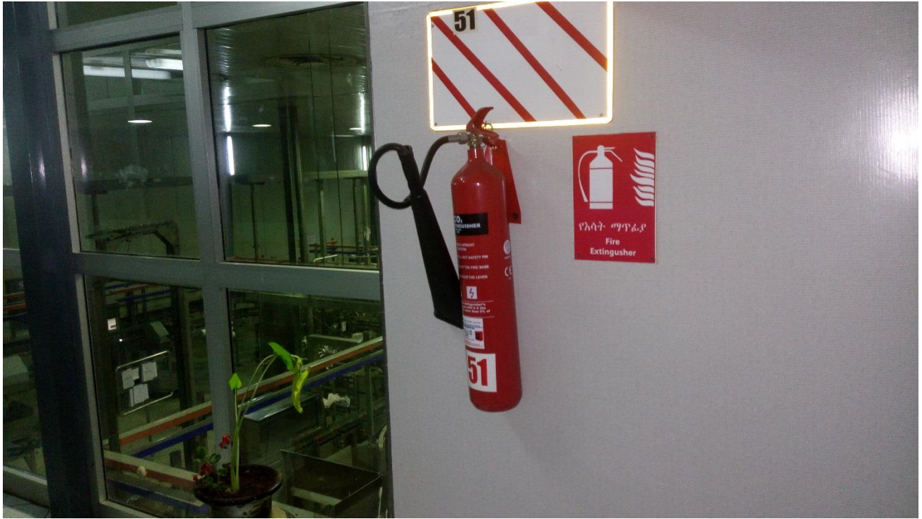
Picture 5 Fire Extinguisher in Manufacturing Line
