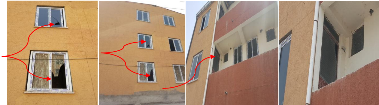
Figure 4.4: Shows defects on door and window mirror broken
