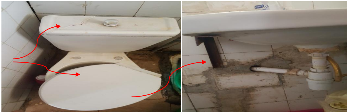
Figure 4.3: Improper sanitary fixtures and broken toilet sink
