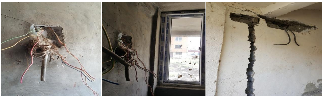
Figure 4.5: Show defects on electrical fittings.
