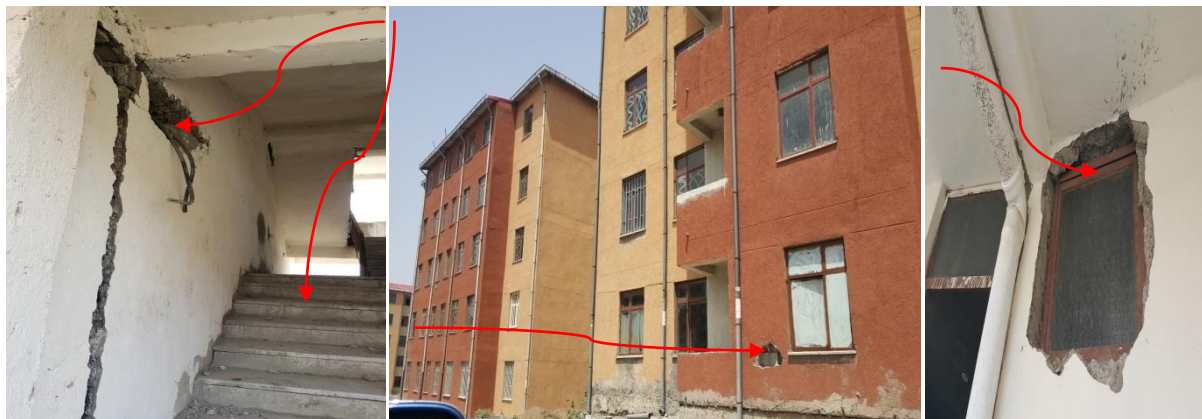
Figure 4.6: Show defects on wall, unfit window and staircases.
