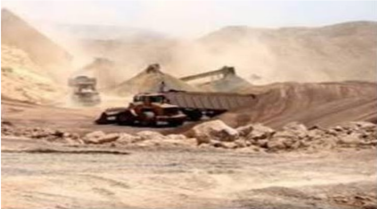
Fig. 4.2 Stone crushing plant in Jimma quarry site
